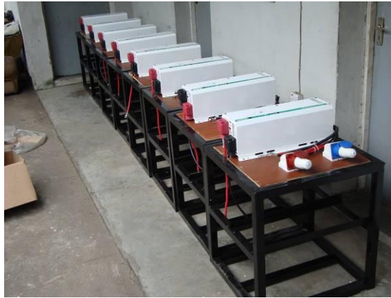
Inverters for a Project
